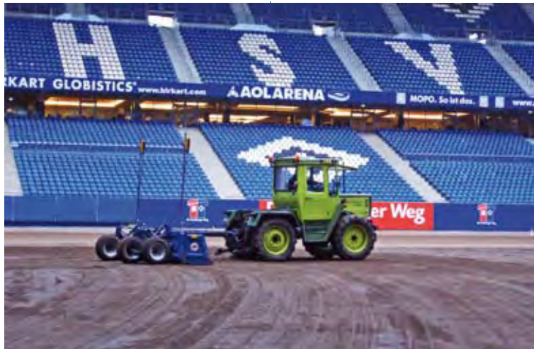
Within four hours the entire surface was planed with a kilver from the Dutch company AP. It has a work width of 2.5 meters and an auto-
